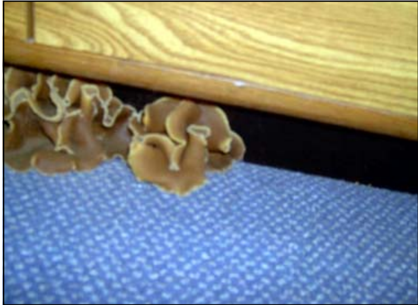
Fruiting bodies of a Peziza sp. in a room with chronic water damage. Peziza sp. is an ascomycete (producing sexual ascospores in a structure called the ascus) and is also known as one of the cup fungi. It is occasionally found on chronically wet or water-damaged wood products (such as plywood subfloor). Peziza can be identified only when the sexual fruiting body is present. In culture, its vegetative state is named Chromelosporium sp. (Unknown or anonymous author; image courtesy of Dr. Chin S. Yang of P&K Microbiology Services)
